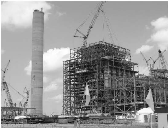
Units 1 and 2 Frontal Views, Late July 2009
